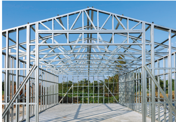
With steel precisely cut and ready to be assembled, less time is needed on the jobsite for fabrication and correcting mistakes.
